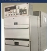
33 KV SF6 PANEL
